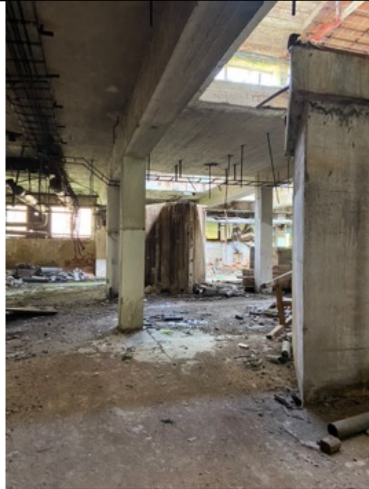
Dyeing works, ground floor, with bases of the dyeing centrifuges. Photos Ivo Hammer 2021
