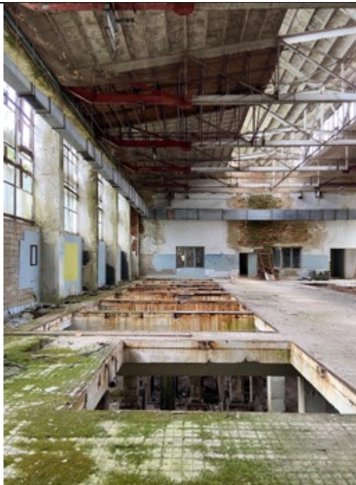
Schindler's Ark, dye works. Reinforced concrete construction with large north windows, facing south, closed towards the annex. Reinforced concrete floor with openings for the centrifuges,
