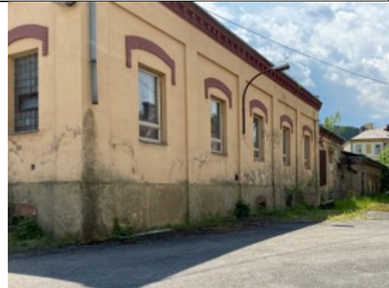
Carding?), View from the northeast. Around 1900? With pilaster strips, segment-arched crowning of the windows, profiled brick eaves with tooth cut, smooth (cement?) Plaster, whitewashed yellow. Flat roof. Crowning the east facade. Photos: Ivo Hammer 2021
