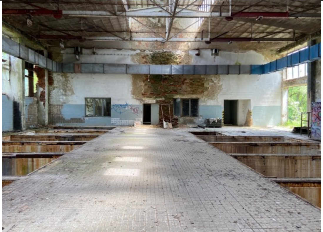
Schindler's Ark, dye works, looking east. Concrete tiles of the floor with wedge joints. The steel structure of the roof with ribbon windows opening to the north and south. Photos: Ivo Hammer 2021
