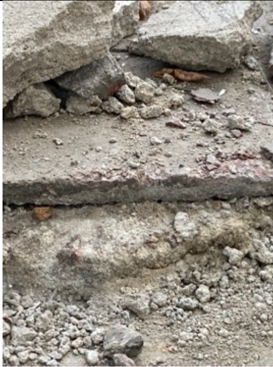
Spinning mill from approx. 1890, northern interior, broken edge of a machine pit: Under the destroyed recent concrete messenger, a possibly original slab of red terrazzo. Photo: Ivo Hammer 2021
