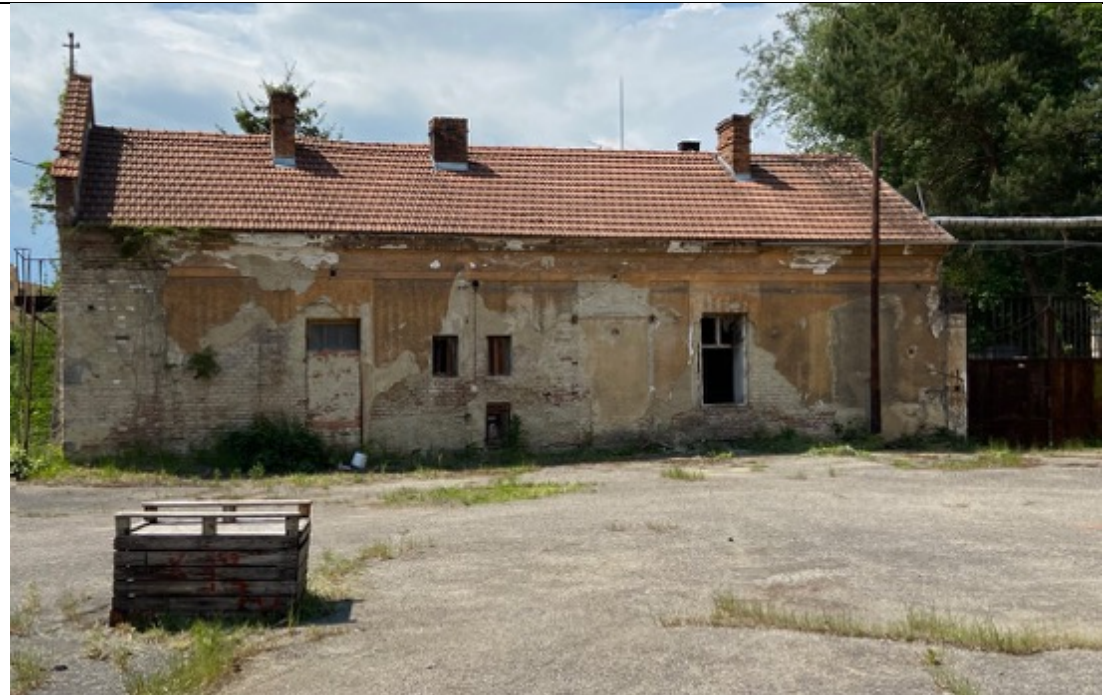
Residential building (management by Oskar and Emilie Schindler). Brick, block bond. Profiled eaves cornice. Raised south gable. 3 (?) Chimneys. Walled up doors. A window walled up with cement mortar. Photos: Ivo Hammer 2021
