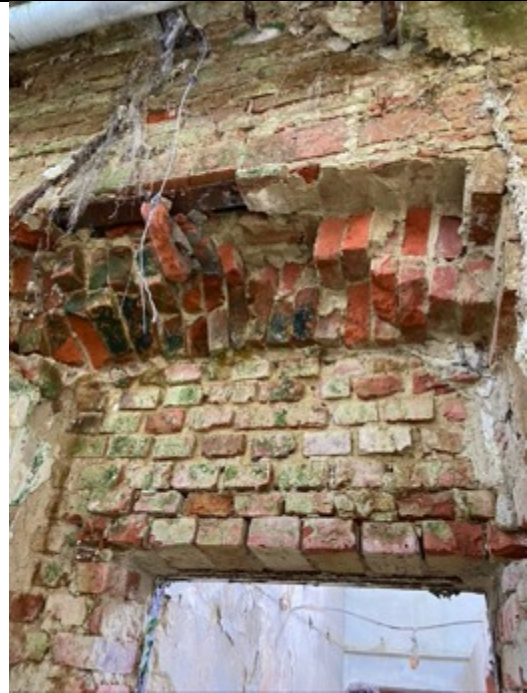
Spinning mill from around 1890, northern interior, east wall, detail. The brownish masonry mortar is visible on the broken-out segmental arch overlay of the door. Photo: Ivo Hammer 2021
