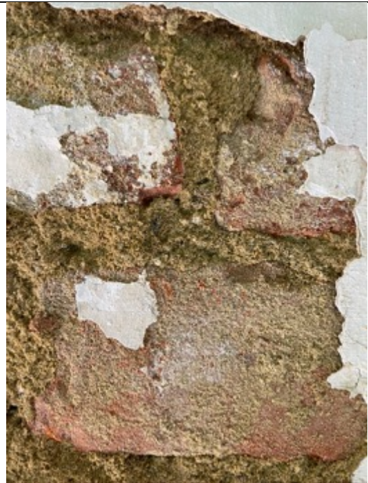
Schindler's Ark, 2nd floor, reinforced concrete hall, northern annex room, view to the south, detail: bricks, brownish masonry mortar, yellowish white lime whitewashes. 1-2 later whitewashes. Photo: Ivo Hammer 2021
