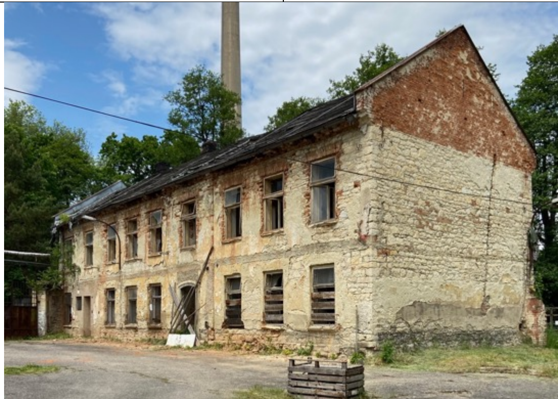
Former laboratory and workshop (SS-Bau des KZ Brnenec, German building). 2 construction phases: stone masonry mixed with bricks, 2 storeys. Gable wall built with brick. The windows on the upper floor possibly enlarged with brick, with a wedge-shaped brick lintel. Both gable walls raised. 2 chimneys in the east. Roof covered (2012?), Only the roof battens left. Completely devastated inside. Remains of plaster and whitewash preserved on the south facade. Window frames and window sashes still partially preserved. Photos: Ivo Hammer 2021
