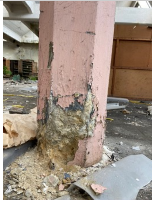
Spinning mill from approx. 1890, south interior, detail of a pillar. The cement is the brownish Roman cement. A touch up? Photo: Ivo Hammer 2021
