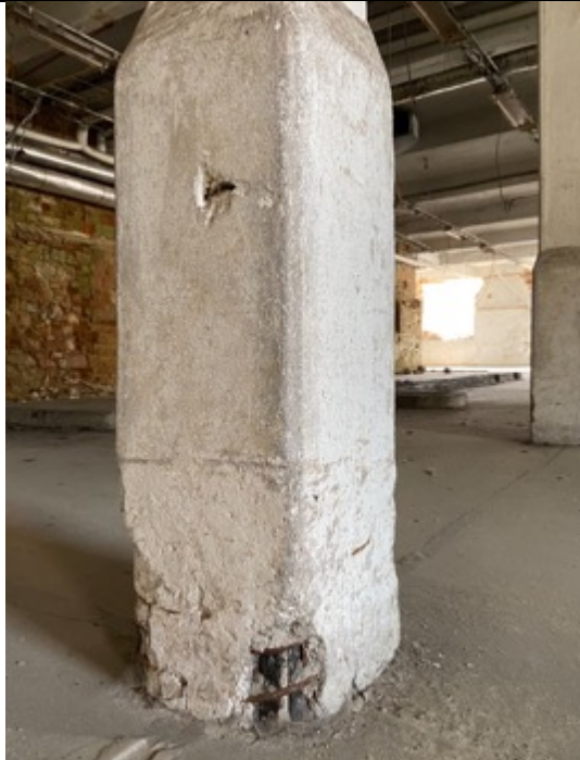
Schindler's Ark, 2nd floor, reinforced concrete hall, view to the southeast, detail: reinforcement of the pillar with reinforced concrete. Photos: Ivo Hammer 2021
