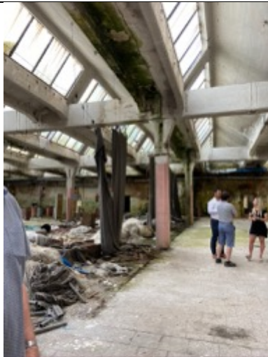
Spinning mill from approx. 1890, northern interior, joint between two yoke compartments in the side member and the cross member. In this area, the pillar is not monolithically connected to the girders. Photo: Ivo Hammer 2021
