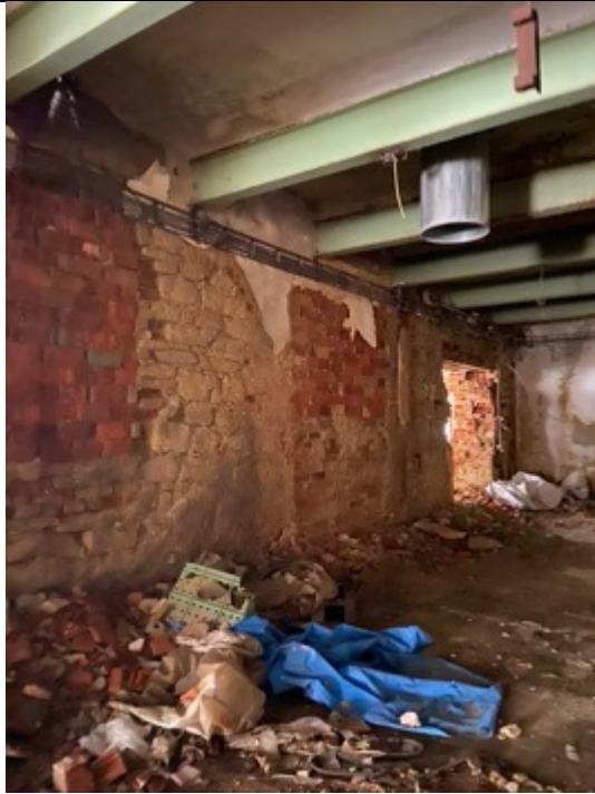
Schindler's Ark, ground floor, room east of the reinforced concrete hall. Stone masonry rebuilt with bricks.
