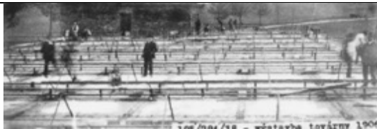
Construction of a weaving hall (Moses Löw-Beer company) in Ingrowitz (Jimramov-Benátky), 1906. Photo from PS 2017, p. 125 (Pavel Novotný archive)
