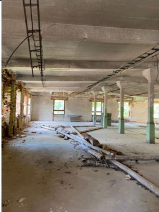
Schindler's Ark, 2nd floor, reinforced concrete hall, view to the south. Photo: Ivo Hammer 2021
