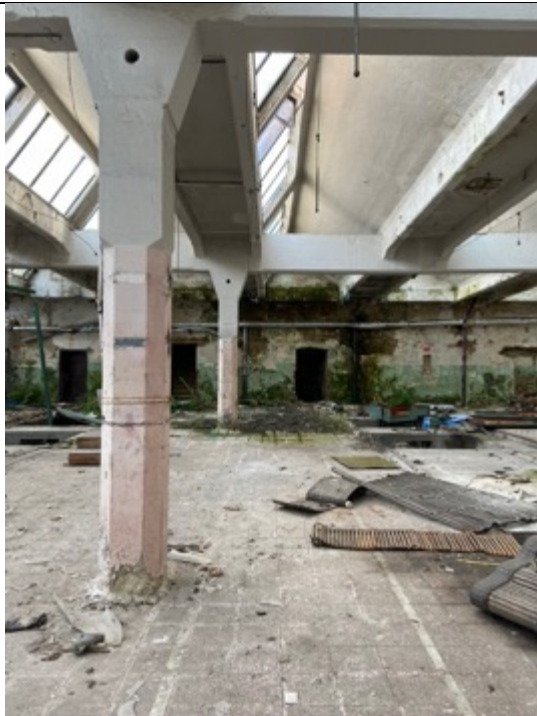
Spinning mill from approx. 1890, north interior, view to the east. Photo: Ivo Hammer 2021
