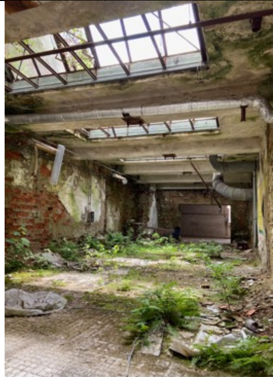
Schindler's Ark, 2nd floor, space between the reinforced concrete hall and the dye works, view to the southeast, reinforced concrete ceiling with hypäthral light.
