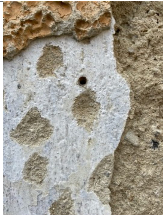
Rubbed surface, very light yellowish-white, thin Freko whitewash. 2 thin yellowish-white whitewashes. Stubby plaster with light gray mortar with fine lime sparrows, possibly natural plaster 3 whitewashes: brown, light red-brown, green. Photos: Ivo Hammer 2021
