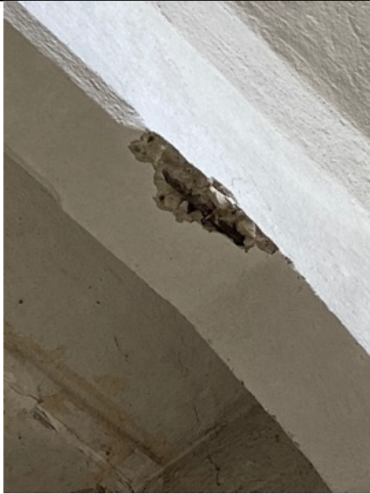
Spinning mill from approx. 1890, northern (?) Interior, detail of a cross member. The gray cement mortar and the reinforcing iron are visible in the mechanical damage. Photo: Ivo Hammer 2021
