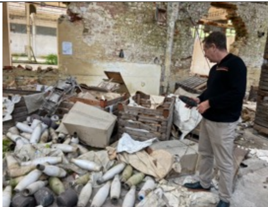
Spinning mill from approx. 1890, southern interior, devastated in 2012 (?). Daniel Low-Beer with the rest of a fabric product. Photo: Ivo Hammer 2021
