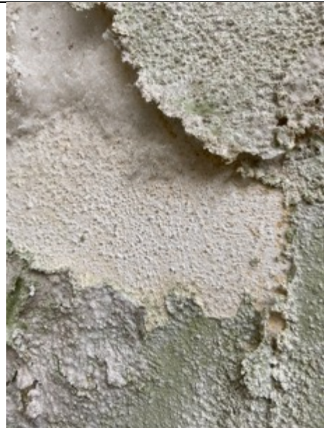
Spinning mill from approx. 1890, northern interior, detail of the west wall. Possibly original rubbed and whitewashed surface. Photo: Ivo Hammer 2021
