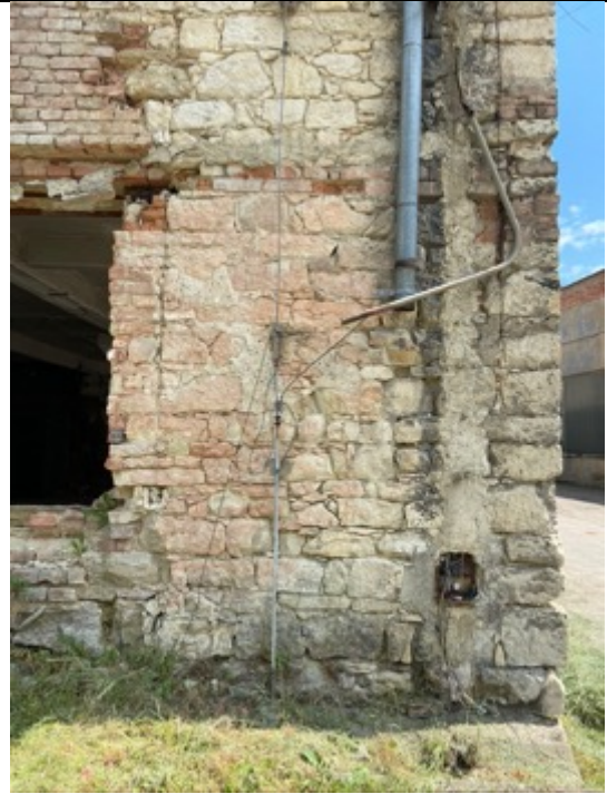
Local pink discoloration of the stone from the source of the fire.
