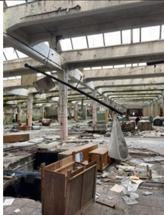
Spinning mill from approx. 1890, northern interior, machine pit and the rest of the heating pipes below the cross member. Photo: Ivo Hammer 2021
